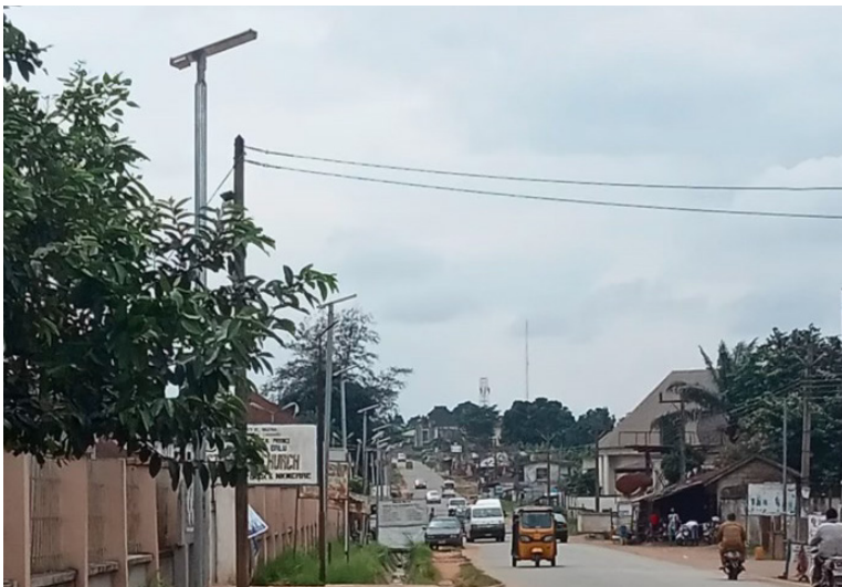
i Installed solar streetlights in Amaigbo community, Imo State
