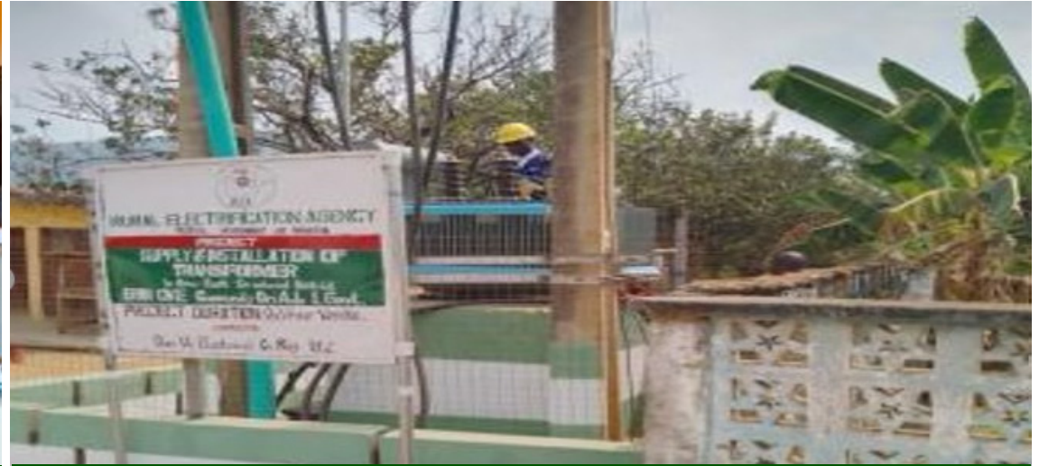
i Transformer installed in, Ekiti State
