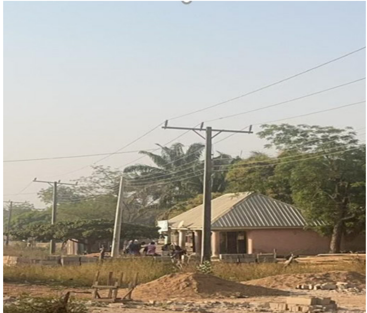
i Distribution lines deployed in Ajewanle, Ilorin, Kwara State
