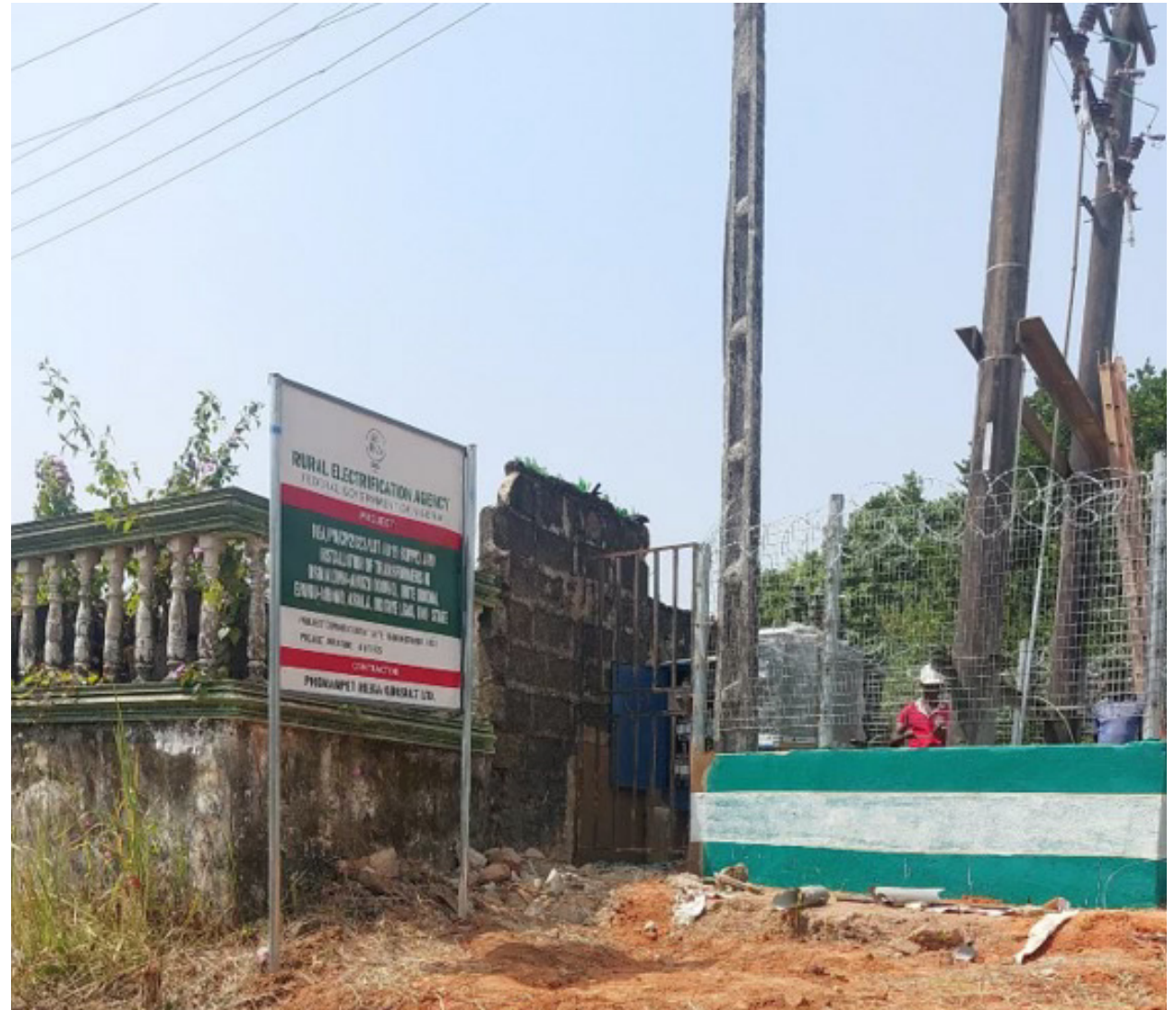
i 300kVA, 33/0.400kV Transformer deployed in Okigwe Local Government Area, Imo State
