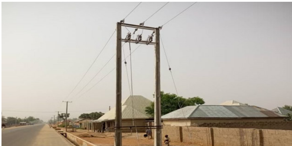
i Installation of 300kVA, 11/0.400kV Transformers, 1km HT Conductor and 2.8km LT Conductor in Yola South LGA, Adamawa State
