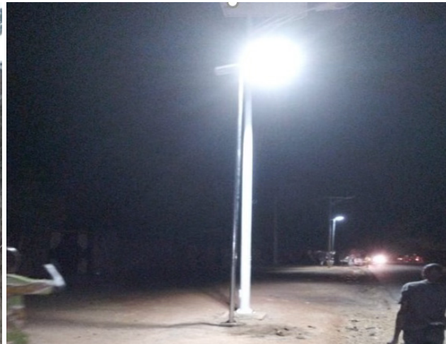
i Installation of 60Watts integrated Solar Streetlights in Mayo Bani, Borno State
