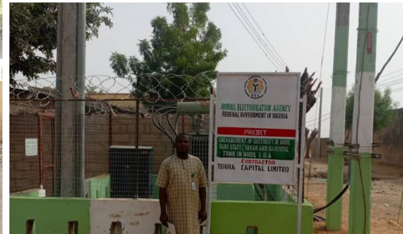
i Transformer installed, serving the residents of Wudil, Kano State
