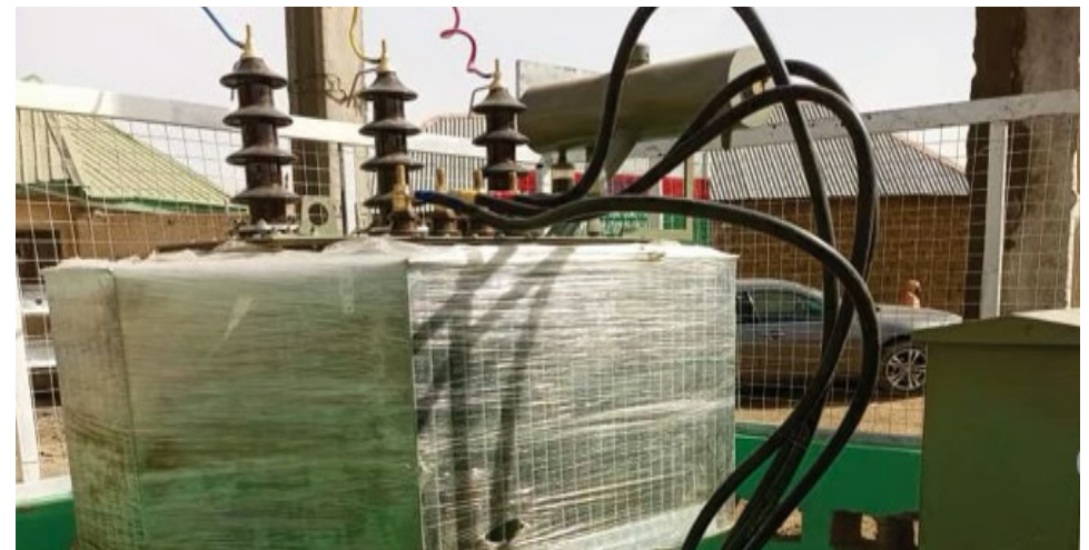
i 300KVA, 33/0.415kV Transformer and LT Reticulation in Boto, Bauchi State
