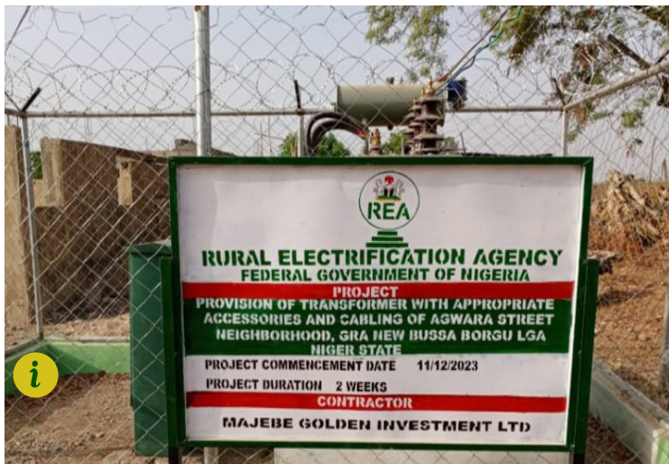
i 300kVA,110.415kVA Transformer Powering Agwara, New Bussa, Borgu LGA, Niger State
